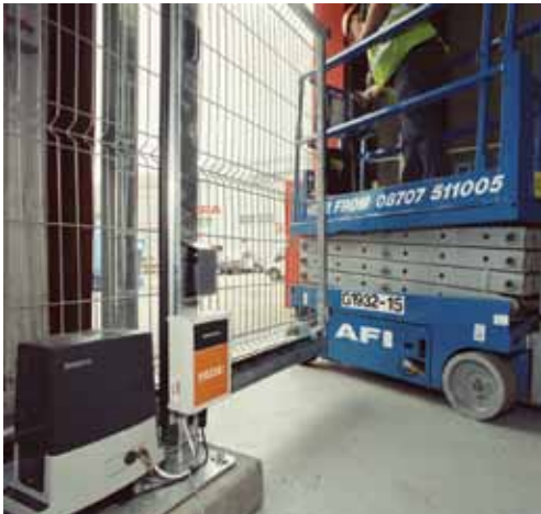
The new system controlling gate access to a site.
